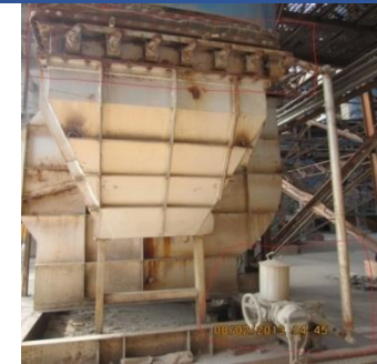
Before: All bag filter fans in DOL Operation
